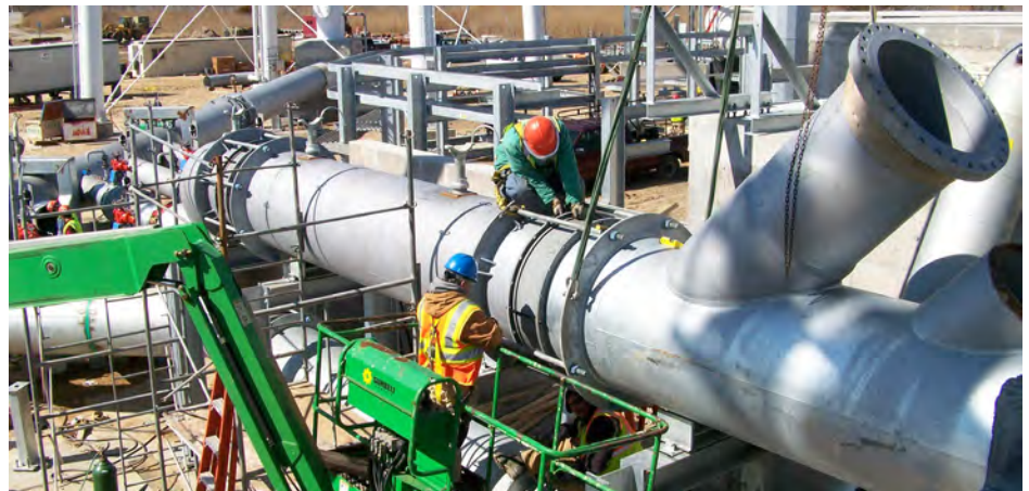
The Sauer Group relied on custom-built pipe slide assemblies—Anvil Figure 439s—to support the deluge piping system as it branched off of the launch pad water tower. The slide assemblies were attached to structural frame supports.
