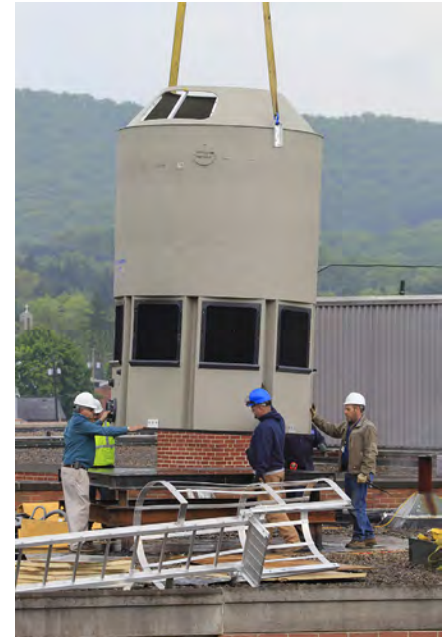
Delta Cooling Towers' advanced plastic cooling towers met the rigorous demands of Davis Memorial Hospital for high performance and minimal maintenance while also providing quieter, more energy-efficient operation.
