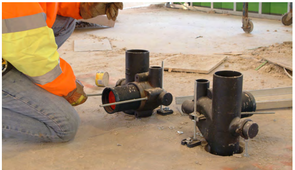
Chad Krajewski, MLP plumbing foreman, installed the Zurn Z1209-F Water Closet Carrier, in a Buffalo, NY, nursing home—one of many Zurn products that helped MLP keep installation time to a minimum.
