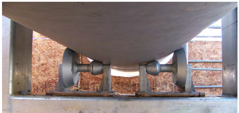
Sauer Group employed Anvil's Figure 76SD fabricated roller for large-diameter pipe and custom-built Anvil Figure 439 structural H slide assembly, shown here, to support the deluge system pipe for the launch pad water tower.
