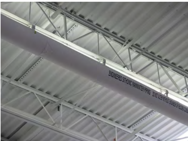
Mercy Hospital used the Wade HydroMax siphonic roof drainage system where the pipework ran completely flat, so it did not need to be installed in the ceiling, which was already congested with traditional and hospital-specific building components.
