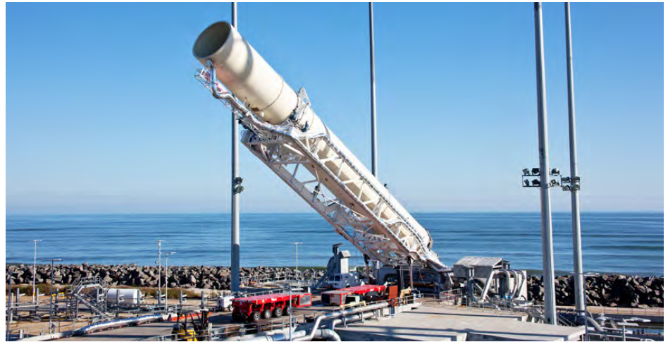
The Sauer Group used Anvil pipe supports and rollers to create the support structure for the 307-foot water tower—the world's tallest launch pad water tower—at NASA's Mid-Atlantic Regional Spaceport.
