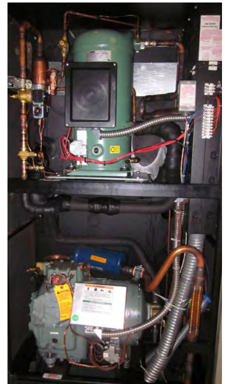
Industrial Cooling Corporation retrofitted a 10-ton reciprocating compressor with a BITZER scroll compressor to keep overall client costs down, reduce power consumption, and minimize noise.
