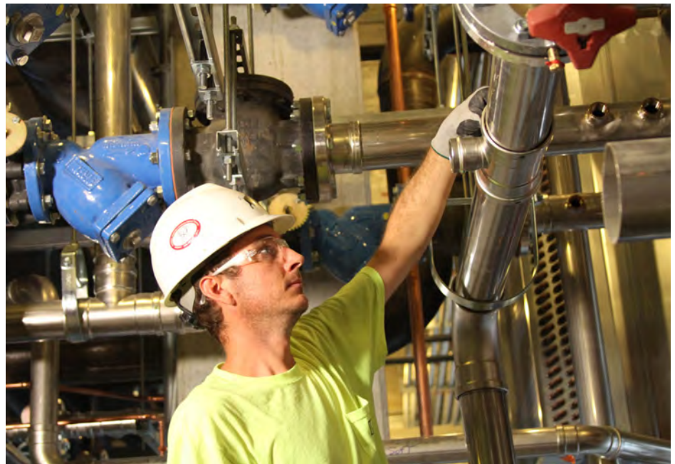
Nelson Stark chose Viega ProPress for stainless steel for the cost savings for the Mercy Health—West Hospital. Using ProPress and prefabrication shortened the installation time and saved labor costs.
