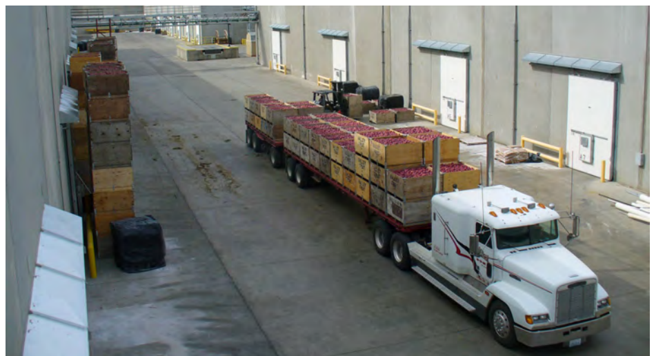
Doubl-Kold bought several hundred tons of BAC's VCA evaporative condensers to increase cold storage capacity for Washington's apple orchards during a record harvest in 2012. Doubl-Kold anticipates a 20-percent increase in the need for cold storage this year as Washington apple exports continue to rise.
