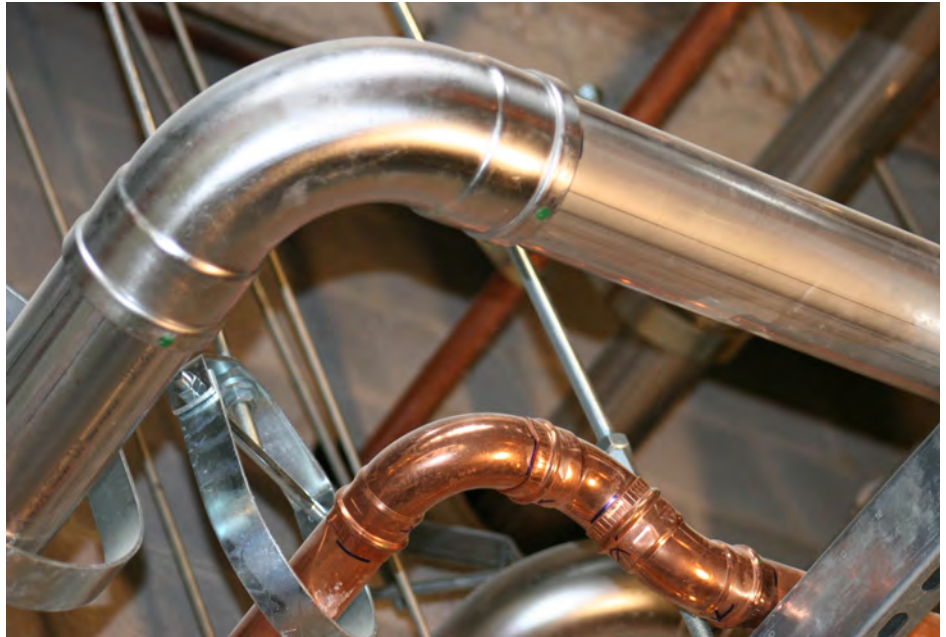
Nelson Stark Company is installing thousands of feet of Viega ProPress systems for both copper and stainless steel at Mercy Health—West Hospital. Having one tool that can press both types saves time and labor.
